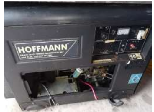
5Kva diesel generator - Fuel pump issues R3500
